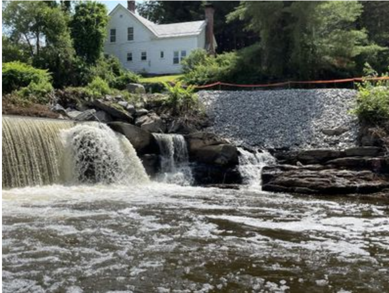
Left abutment/training wall scour and temporary repair for roadway
