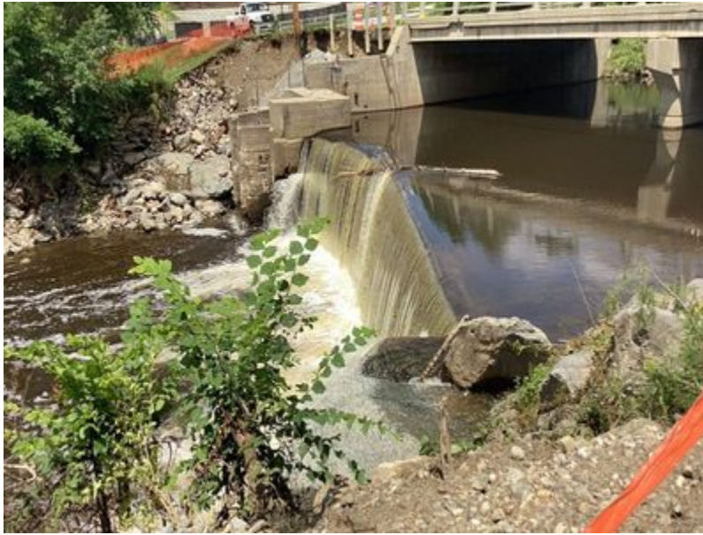
Overview of spillway with abutment scour from left abutment
