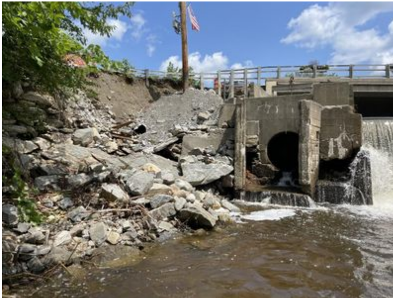
Right training wall/abutment scour after VTrans material placement
