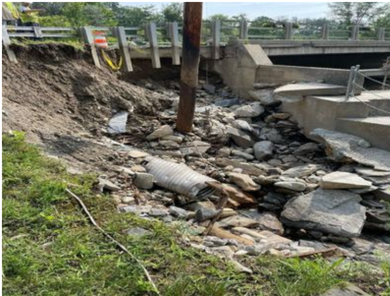
Scour along right training wall/LLO. Photo provided by Shane the Town Administrator from before VT Trans temp fill
